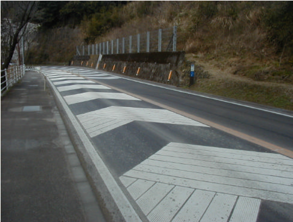
Chevron Sign Marking (anti-skid type)
